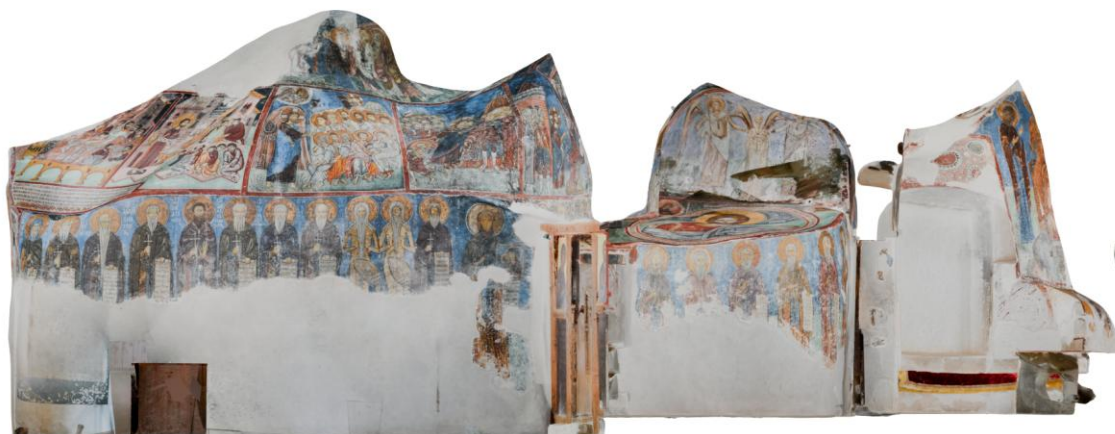
Internal Orthographic Cross Section at the central horizontal axis towards the east wall of the Enkleistra
